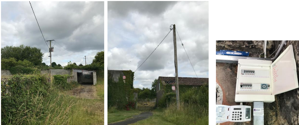
Figure 4. Existing above ground electricity lines feeding Wonderful Barn
